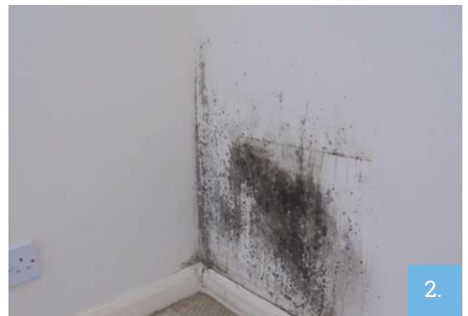
Condensation mould in the corner of a room exposed after furniture removed.
